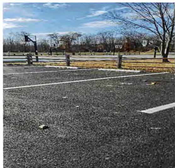
Adjacent Parking Area with Lines and Blocks
