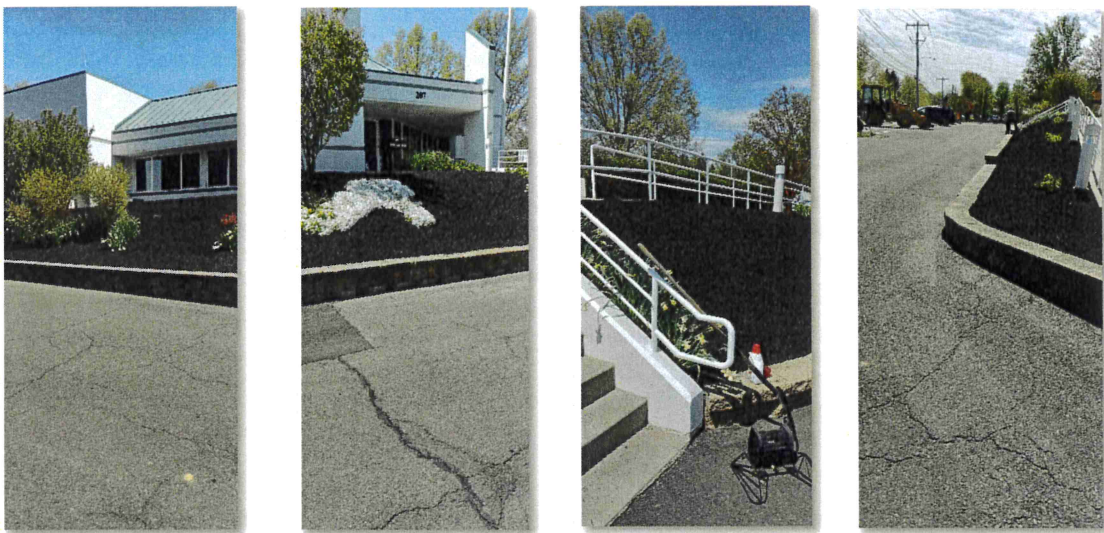
All Above Pictures are the Finished Result at the Front of Administration Building
