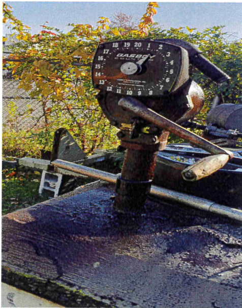
Old Pump With Obvious Leaking Issues
