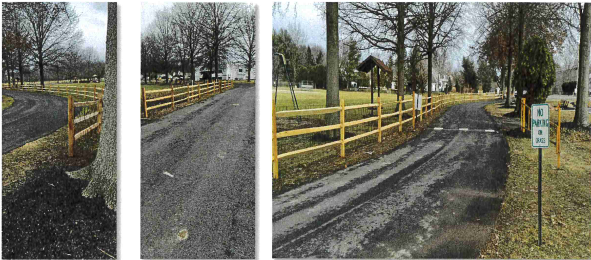
View of newly installed fence at North Branch Park along the main entrance to Pavilion #1
