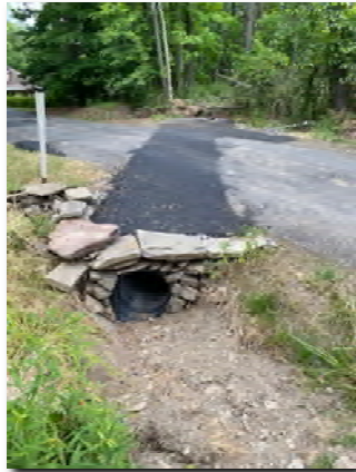
Chapman Rd. Cross Pipe
